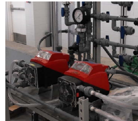
Chemical Dosing Pumps
